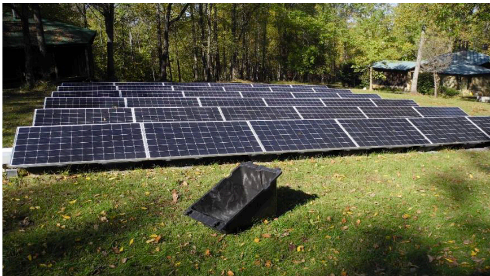
Figure 2. PowerField PV Solar Array
