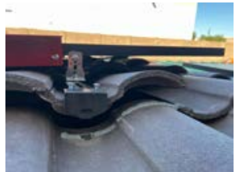
PHOTO 9: Bracket unloaded after test - roof tile bond pulled apart.
